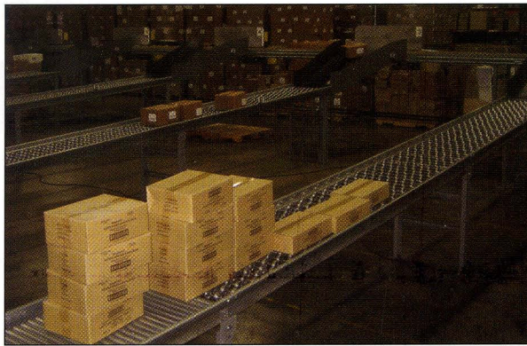
Sergeant's Pet Care Products automated its picking process by installing a conveyor and swing-arm sorter from TGW-Ermanco (Spring Lake, Mich., www.tgw-ermanco.com ), and warehouse control software from Tech King.
